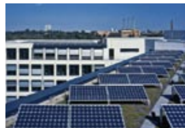
PV-Light flat-roof construction with a total output of 20 kWp
