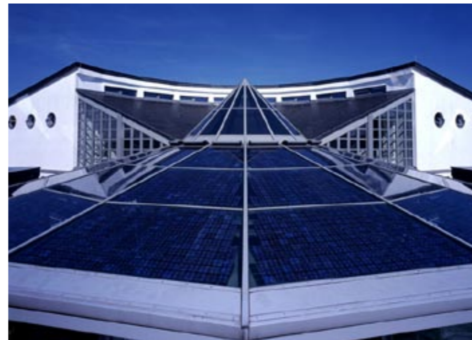
Aluminium skylight construction – external view. 60 modules in 20 different sizes with a total output of 11 kWp
