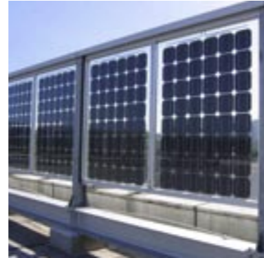
Bifacial photovoltaic modules, inserted in a free-standing spandrel panel
