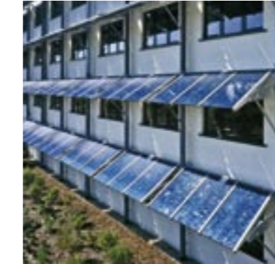
234 frameless modules with a total output of 45 kWp in a special canopy construction
